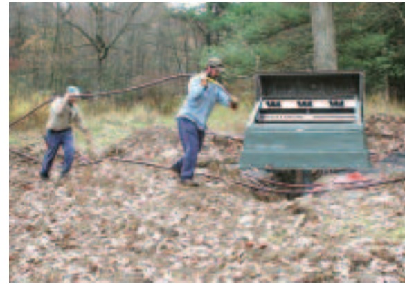
ELECTRIC WORK UNDER WAY: Gary Lafferty and Al Hileman prepare to splice lines at a junction box as part of the new construction project at White Sulphur Springs.
