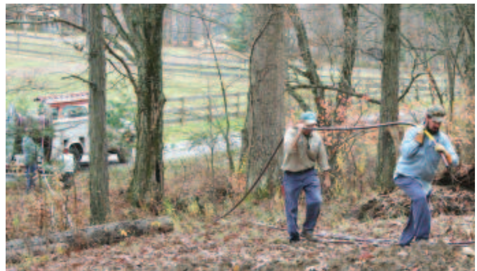
PREPARING FOR EXPANSION: Gary Lafferty and Al Hileman pull one of the four electric service wires through the woods and over a creek in preparation for the service lines for the new building. There are four lines, one a spare, 485 feet in length. Tim Mellott pulls the wire off the reel at the truck.
